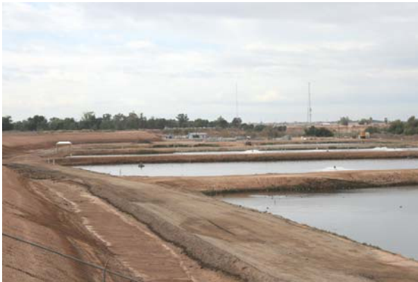
Waste Water Treatment Plant
