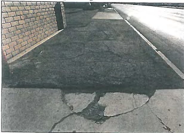
While some sidewalks need repair...
